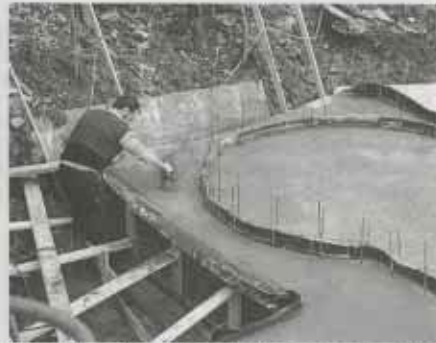
Smoothing the surface of the concrete prior to extending the waterproofing layer.
