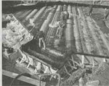
Laying the waterproofing directly on to the concrete bed followed by the protective concrete layer.
